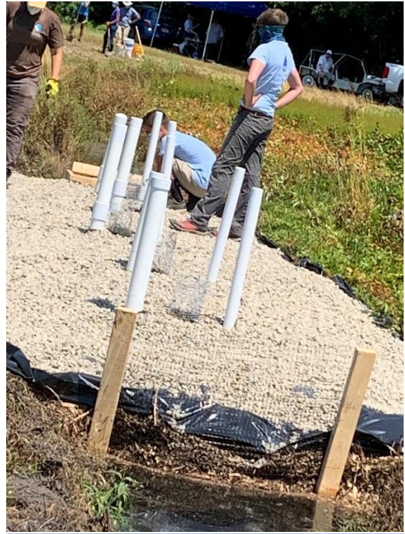
Completed bioreactor installation in Marstons Mills, Massachusetts in July 2020
