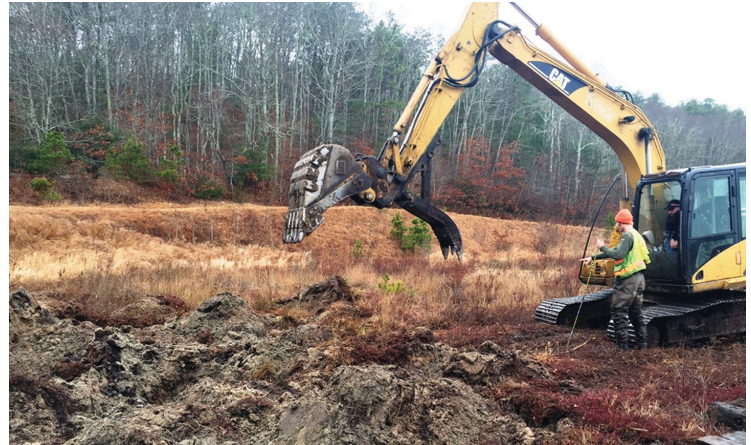
Layers of sand and peat are dug up during construction of cranberry bog restorations, encouraging the growth of vegetation.
