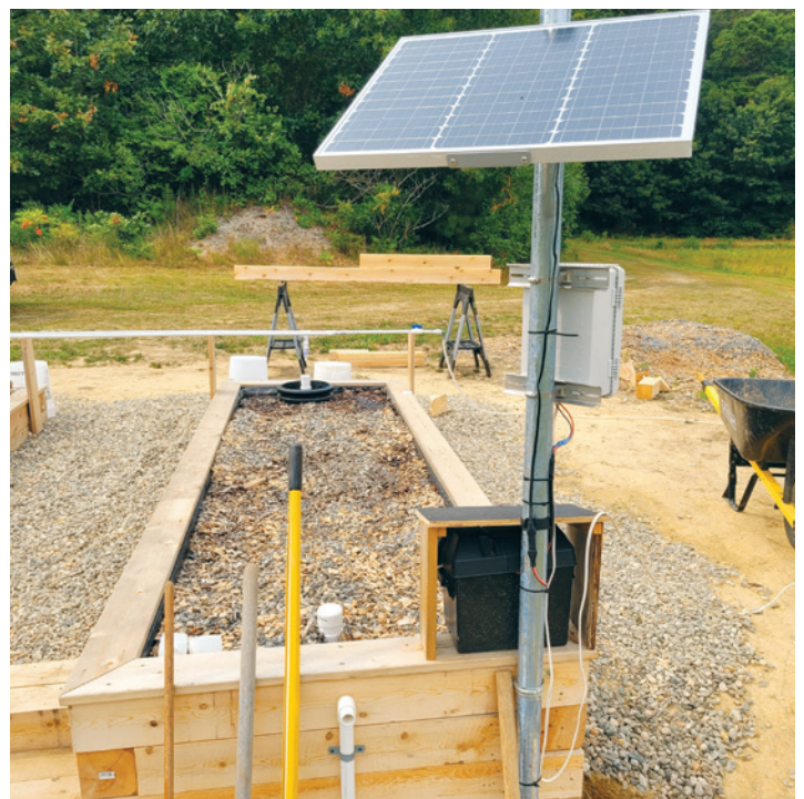
Woodchip/Stone bioreactor with solar power panel.
