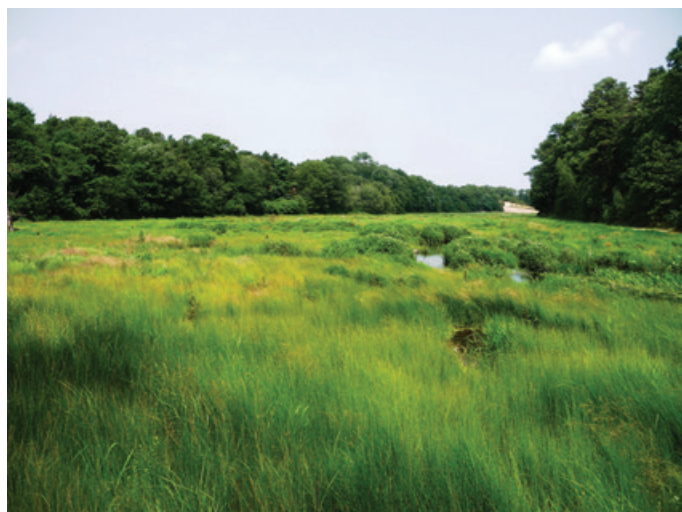
Four months after construction began, plant growth can be seen along a reconstructed stream channel. (2010)
